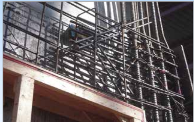
Accurate simulation allows visualization for review of reinforcement and embeds helps plan through congestion issues and can be used in the field for placing.
